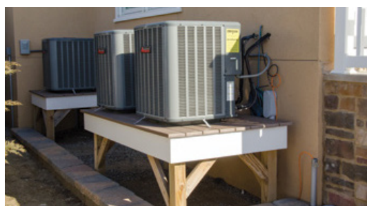
← Elevated equipment Image Credit: FEMA, Liz Roll
