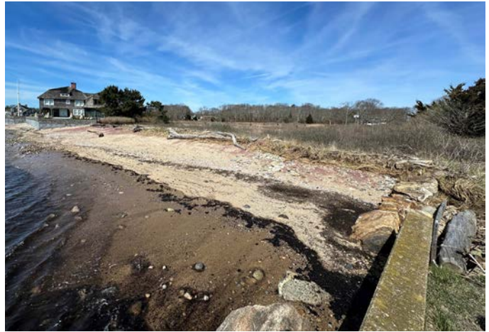
↓ Scum Beach Seawall Gaps - Fenwick
