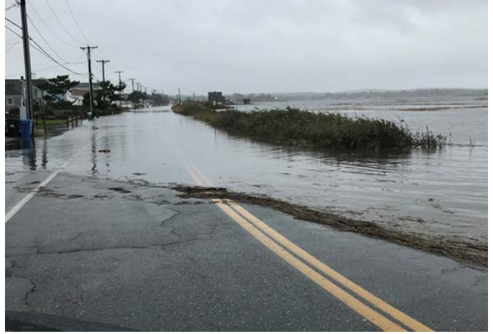
Plum Bank Rd Flooding - Old Saybrook
