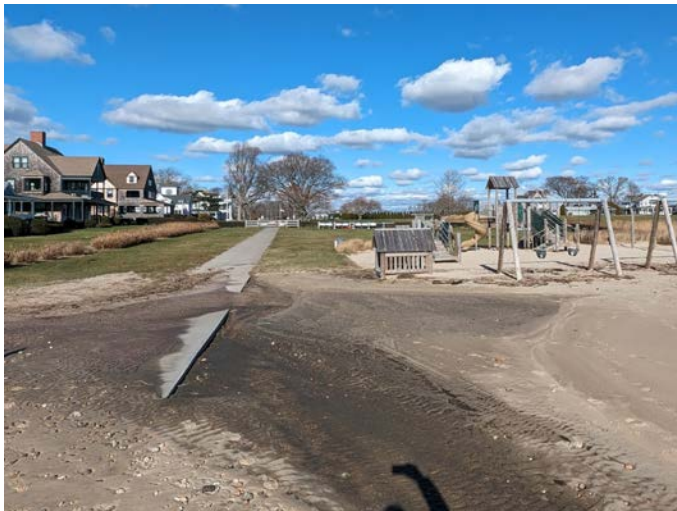
↓ Sand Displacement and Erosion - Fenwick
