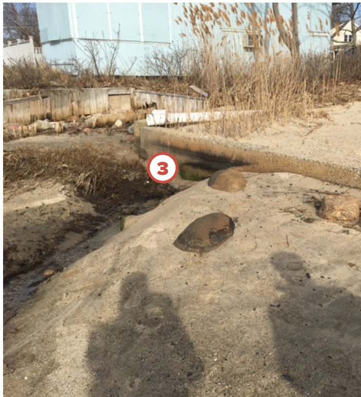
⬆ Existing condition of the outfall between Old Sea Lane and Hartford Avenue.
